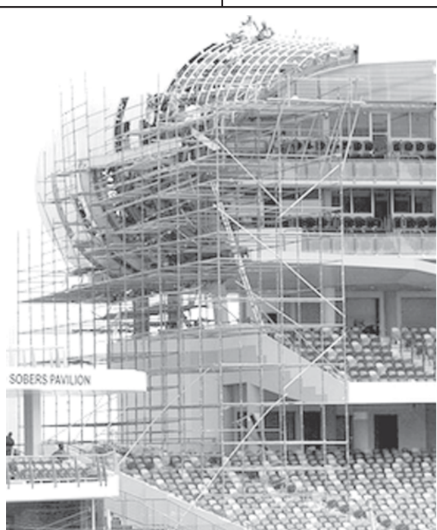
The Worrell, Weekes and Walcott Stand is seen under construction at the Kensington Oval, Bridgetown, Barbados, Tuesday 6 March, 2007. The Kensington Oval, with an enlarged capacity of 28,000, will host the final of the Cricket World Cup on 28 April. — INTERNET
