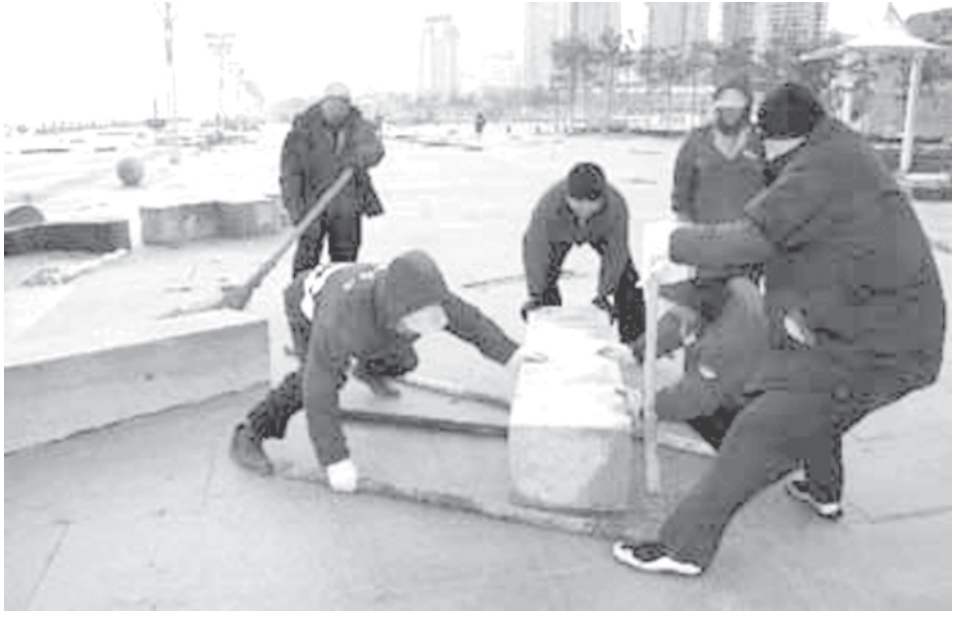
The seashore levee was destroyed by the storm tide in Yantai, a coastal city in east China's Shandong Province, on 4 March, 2007. — XINHUA
