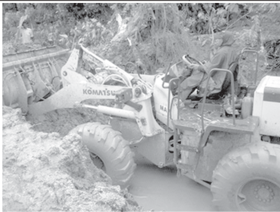
A worker uses heavy equipment to clear mud from a road leading to the site where a landslide killed at least 32 people in Ruteng, Manggarai district, on 3 March. Rescue teams have been sent by air to help find dozens of people still missing after deadly landslides buried villages in eastern Indonesia. —INTERNET
