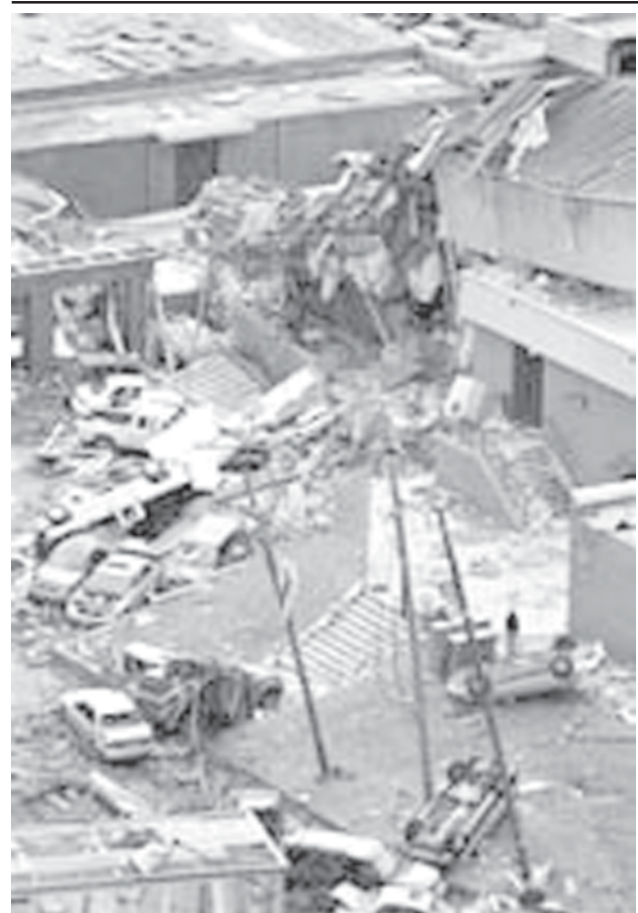
Damage from Thursday's tornado at Enterprise High School is shown, on Friday, 2 March, 2007 in Enterprise, Ala. — INTERNET
