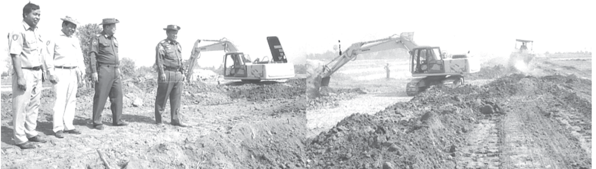
Lt-Gen Ye Myint of Ministry of Defence inspects construction of road linking Yamethin and Tatkon townships. — MNA
