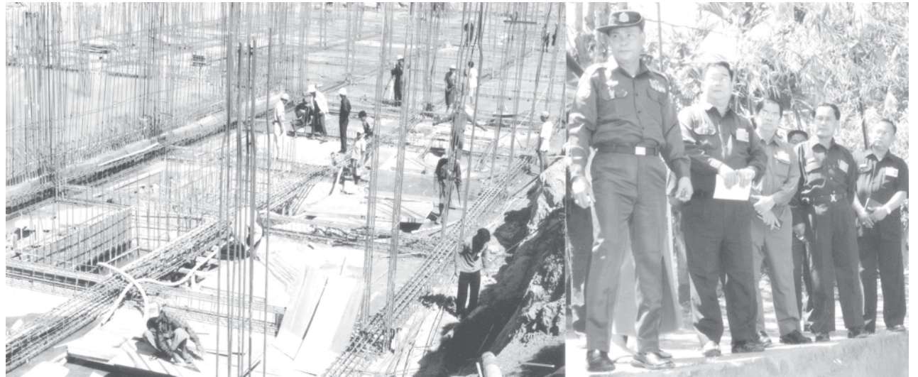
Mayor Brig-Gen Aung Thein Lin inspects construction of tank which will have a storage capacity of 1 million gallons of water in Mayangon Township. — YCDC
