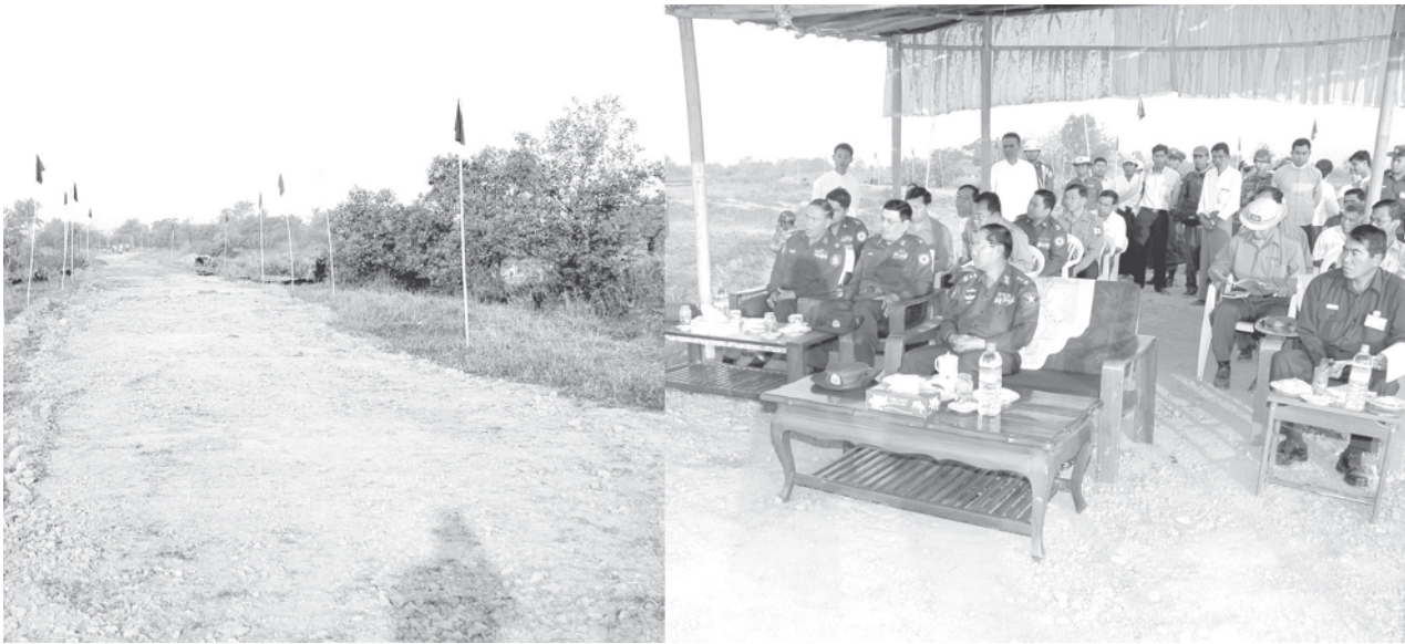
Lt-Gen Myint Swe of Ministry of Defence visits construction of Hlinethaya-Twantay motor road and Tamatakaw-Hteingon-Wayonseik earth Road.
