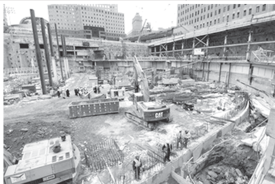
Construction continues on the Freedom Tower with the first planted beams of the left southern edge of the tower visible, on Tuesday, 20 Feb, 2007, in New York. New York Gov Eliot Spitzer visited the site following a news conference in which he announced his support of the under construction tower at the site of the 2001 World Trade Centre. — INTERNET
