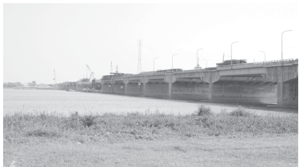
Dagon Bridge linking Dagon Myothit (Seikkan) Township and Thanlyin Township under construction. — MNA
