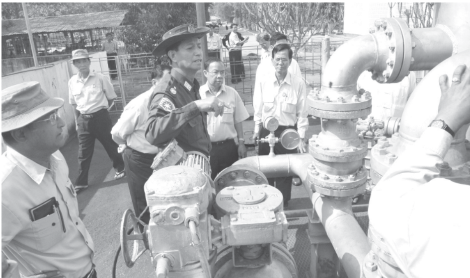
Minister Maj-Gen Khin Maung Myint inspects Thakayta Power Station.—MNA
