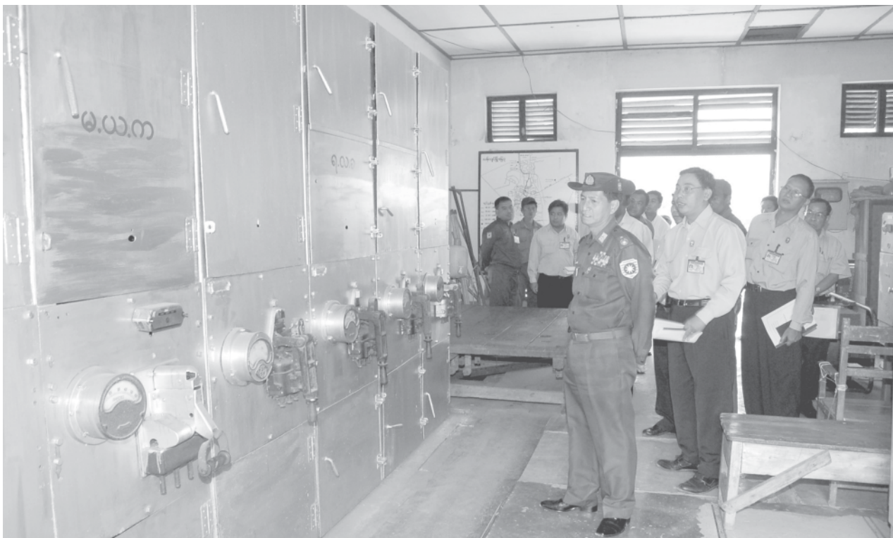
Minister for Electric Power No 2 Maj-Gen Khin Maung Myint inspects Myoma sub-power station in Thanlyin Township. — MNA
