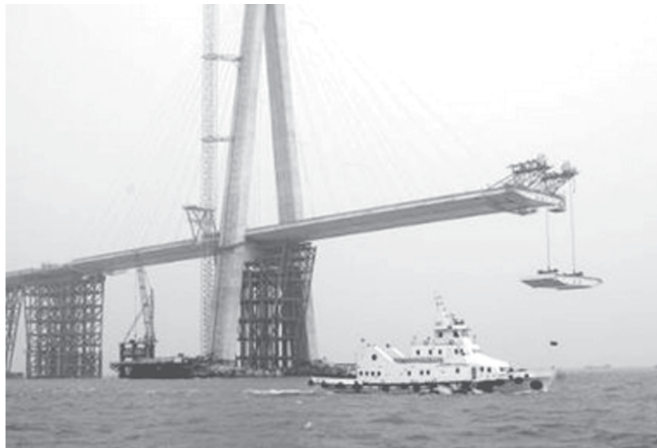
A maritime boat patrols as Sutong Bridge is under construction in east China's Jiangsu Province on 26 Jan, 2007. Sutong Bridge links Suzhou and Nantong in Jiangsu Province, with a main span of 1,088 metres (3,570 ft). —INTERNET
