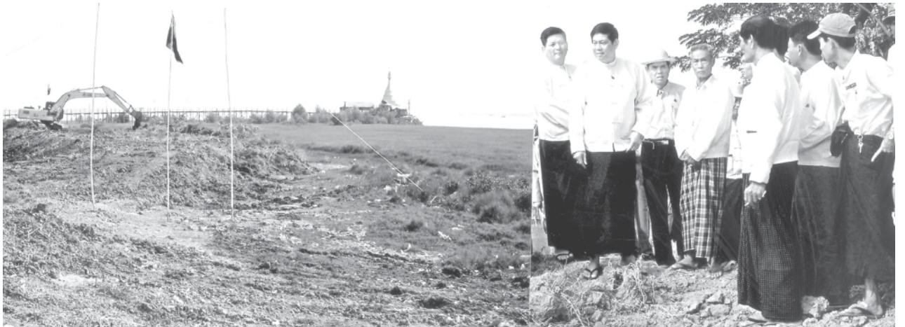
USDA Secretary-General U Htay Oo inspects building of embankment to prevent inflow of salt water to plantations. — A&I
