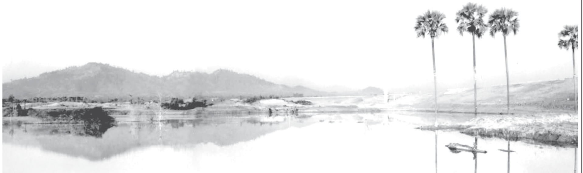
The outfall tower of the Hlaing Chaung Dam in Pale Township, Sagaing Division.
