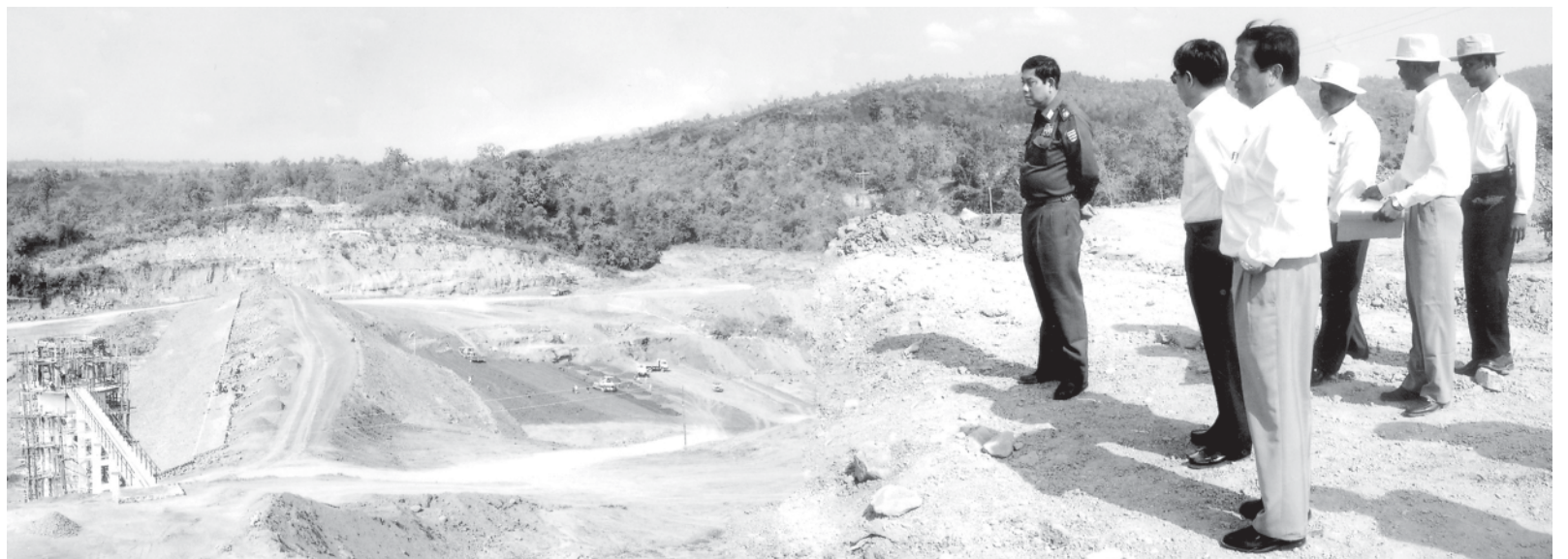
Maj-Gen Htay Oo inspects construction of North Yama Supporting Dam Project in Pale Township. — A&I
