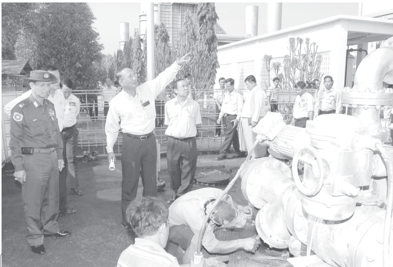
Minister for Electric Power No 2 Maj-Gen Khin Maung Myint inspects laying of gas pipeline. — MNA
