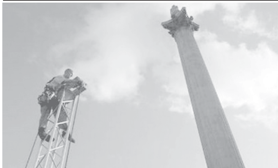
Paul Darby, a rigger, constructs rigging for screens for the New Year's Eve celebrations in Trafalgar Square, London on 30 Dec, 2006. —INTERNET
