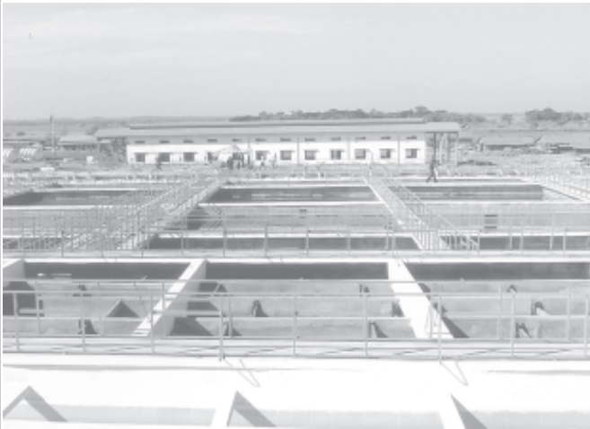
A cluster of tanks under construction to settle sediments carried along the intake canal of the Yangon City Water Supply Project (Ngamoeyeik).
