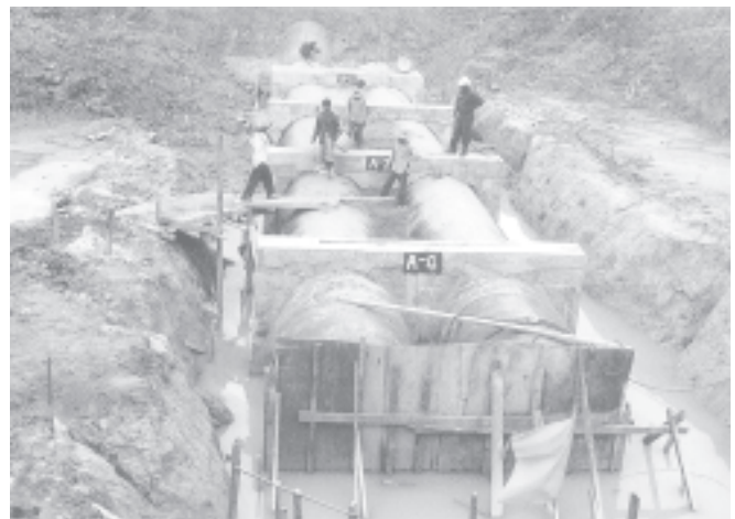
Two 76-inch-diameter steel pipelines being laid to build an intake canal on the bed of the Ngamoeyeik Creek.
