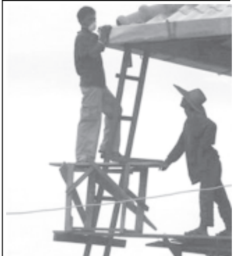
Acehnese men build a new house at Lampuuk village in the outskirts of Banda Aceh, Indonesia, on 24 Dec, 2005. A year after the devastating Asian tsunami, Acehnese are rebuilding their homes and lives, though they are marked by the sadness of losing hundreds of thousands of family members.—INTERNET
