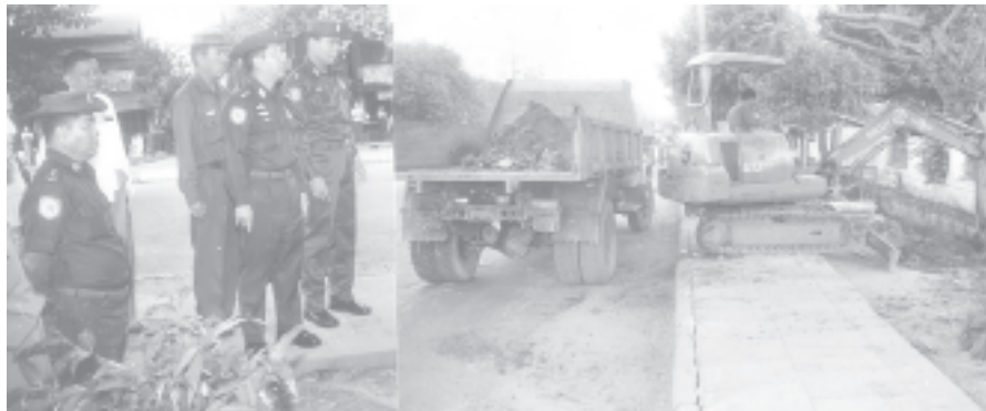
Commander Lt-Gen Myint Swe and Mayor Brig-Gen Aung Thein Lin inspect extended digging of the drain along U Chit Maung Road in Tamway Township. — MNA
