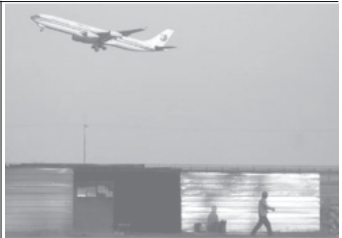
A plane flies over a construction site of Airport Terminal 2 in Pudong International Airport in Shanghai, on 18 Dec, 2005. —INTERNET
