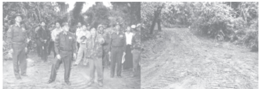
Commander Maj-Gen Ohn Myint and Minister Brig-Gen Thein Zaw inspect construction of the earth road leading to Putao-Phonkanrazi snow-capped mountain.
