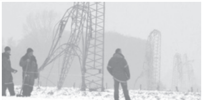
Workers stand in front of damaged power poles in Ochtrop, western Germany, on 28 Nov, 2005. Power poles were bent during a snow storm that caused a blackout in some German cities over the weekend.—INTERNET
