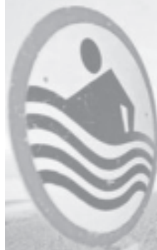
Thai workers install a warning system onto a tower at a beach in Phuket, south of Bangkok on 27 Nov, 2005. —INTERNET
