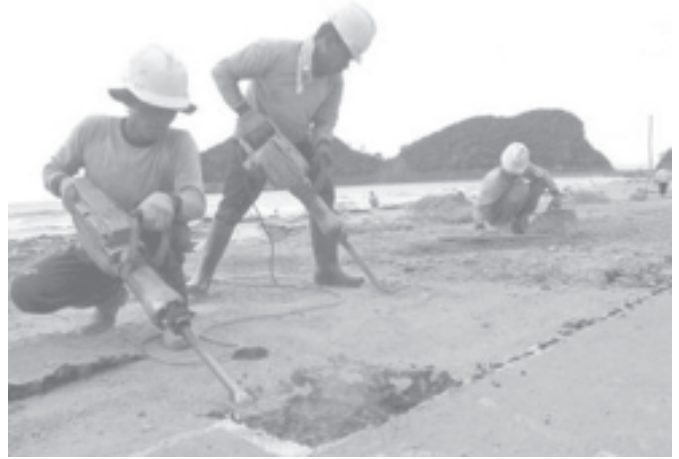
Acehnese workers fix a road in Lhoknga, on the outskirts of the Indonesian city of Banda Aceh, on 26 Nov, 2005, which was devastated by a massive quake-triggered tsunami on 26 Dec, 2004. —INTERNET
