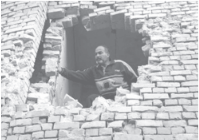
An Iraqi removes rubble from his house after it was damaged by a mortar round explosion in Baghdad on 23 Nov, 2005. —INTERNET
