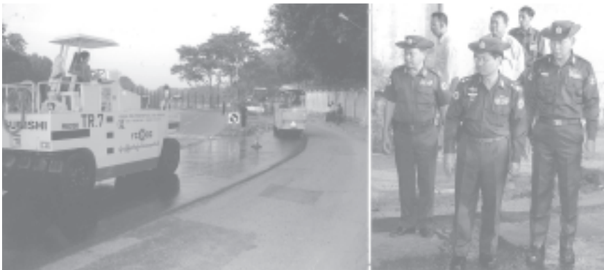
Chairman of Yangon Division Peace and Development Council Commander Lt-Gen Myint Swe and Chairman of YCDC Mayor Brig-Gen Aung Thein Lin inspect tarring of Natmauk Road.
