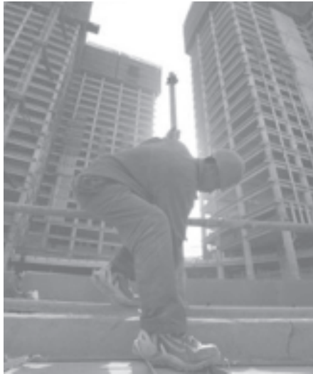
A worker dismantles scaffolding outside a construction site in Beijing on 10 Nov, 2005.
