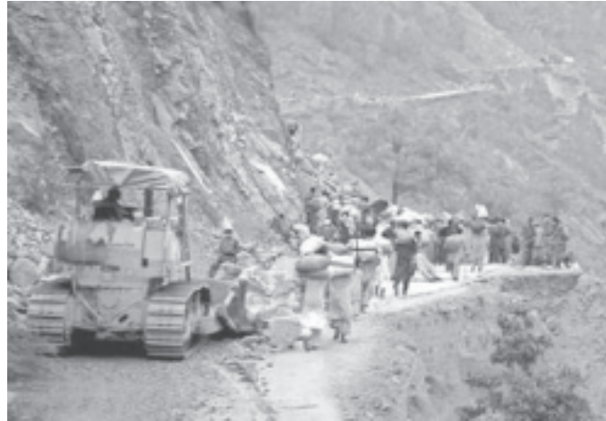
Workers and Pakistani soldiers speed up clearance on the Neelum Valley road, which was heavily damaged by the 8 October earthquake north of Muzaffarabad, the capital of Pakistan-administered Kashmir, about 130km (82 miles) north of Islamabad on 5 Nov, 2005. —INTERNET
