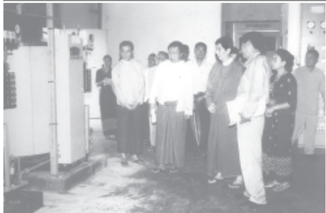
FACTORY INSPECTED: Minister for Health Dr Kyaw Myint inspected Hepatitis-B Vaccine Factory of Medical Research Department (Lower Myanmar) on 23-10-2005. The minister oversees functions of the boiler room of the factory.— HEALTH
