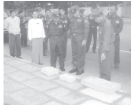
Commander Maj-Gen Myint Swe and Mayor Brig-Gen Aung Thein Lin inspect placing of concrete tiles at platform along U Wisara Road.—MNA
