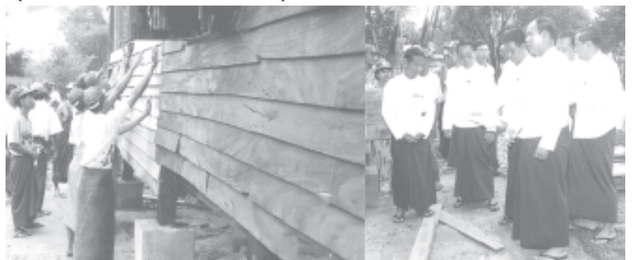
CEC member of USDA Mayor Brig-Gen Aung Thein Lin and party inspect renovation of Basic Education Primary School in Kawhmu Township. —YCBC
