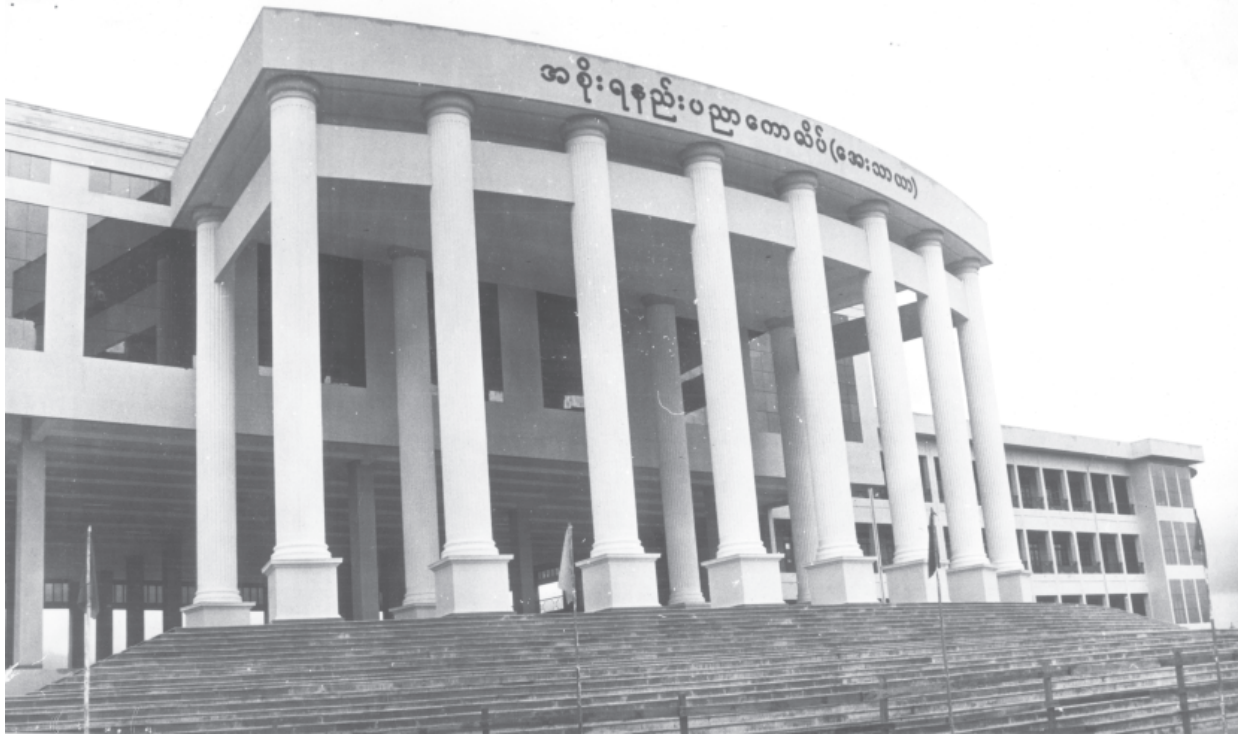
Progress in construction of Government Technological College (Ayethaya) in Taunggyi, Shan State (South).
