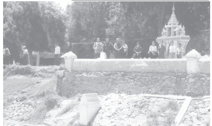
Maj-Gen Kyi Aung inspects construction of embankment to prevent erosion near Sandaku Pagoda in Pwintbyu Township. — CULTURE
