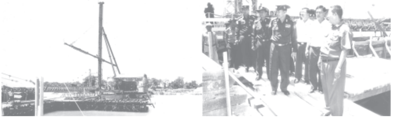
Lt-Gen Khin Maung Than oversees progress in construction of Kyauktan Bridge on An-Sittway Road.— MNA
