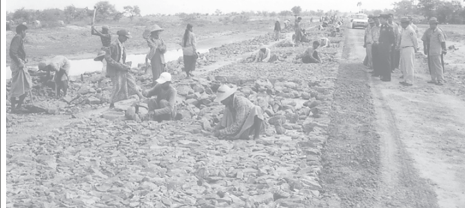
Minister Col Thein Nyunt inspects the construction of district-to-district road No 1 in Mandalay Division on 4-9-2005. — PBANRDA
