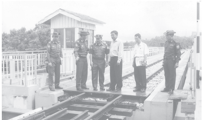
Commander Maj-Gen Soe Naing and Minister Maj-Gen Aung Min inspect the laying of railway lines on Thanlwin Bridge (Mawlamyine). — MR
