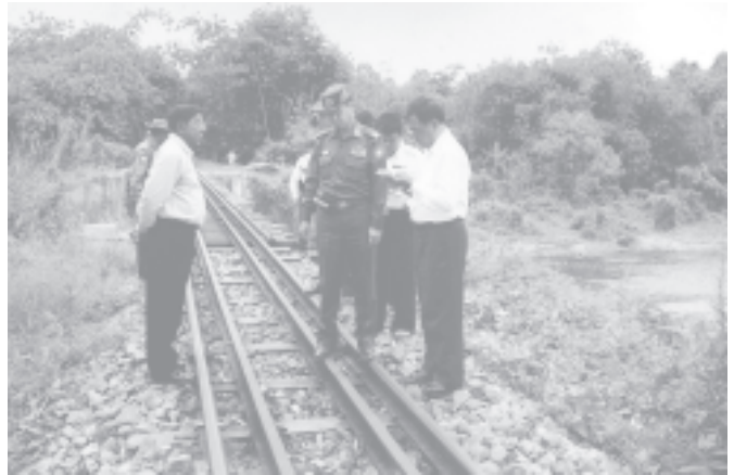
Minister for Rail Transportation Maj-Gen Aung Min inspects Ye-Dawei railroad and gives necessary instructions. — (MYAMNA RAILWAY)
