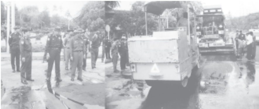
Commander Maj-Gen Myint Swe and Mayor Brig-Gen Aung Thein Lin inspect repaving of Shwegondine Road in Bahan Township.—MNA
