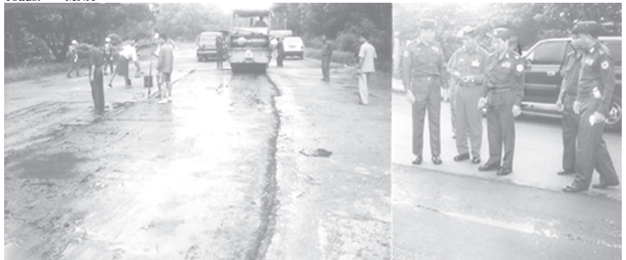
Commander Maj-Gen Myint Swe and Mayor Aung Thein Lin inspect tarmacking of Parami Road in South Okkalapa Township. — MNA
