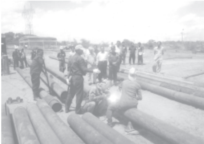
Minister for Energy Brig-Gen Lun Thi inspects laying of new pipeline for Molar CNG Pressed Plant in Chauk.— ENERGY
