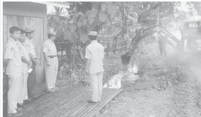
Director-General U Myo Myint inspects tasks for proper drainage in Bago Township.— MNA
