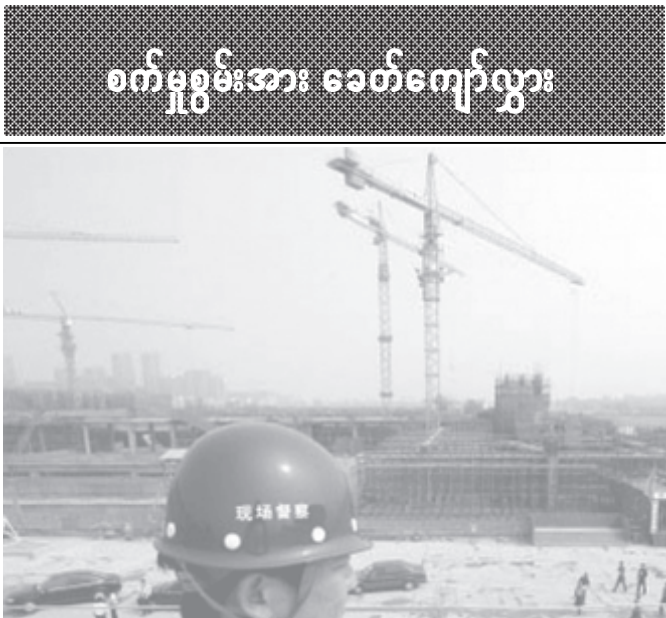
A Chinese guard overlooks the construction site of the Aquatic Centre for the 2008 Olympic Games in Beijing recently. —INTERNET
