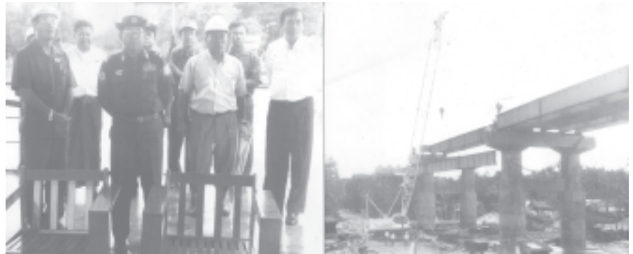
Minister Maj-Gen Saw Tun inspects installation of steel beams at Pyapon Bridge construction site.
