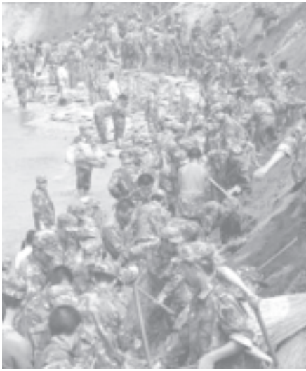
Chinese soldiers repair a section of the bank along the Hunhe River that is damaged by rain-storms in Shengyang, northeast China's Liaoning Province, on 15 August, 2005.
