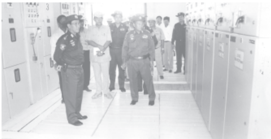
Prime Minister General Soe Win inspects control panel of Inndaw Water Pumping Station Project.—MNA
