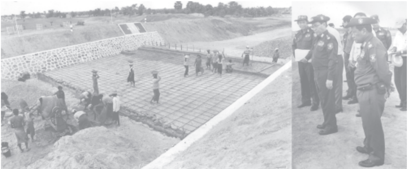
Prime Minister General Soe Win inspects construction of the spillway of Innbat Dam. — MNA
