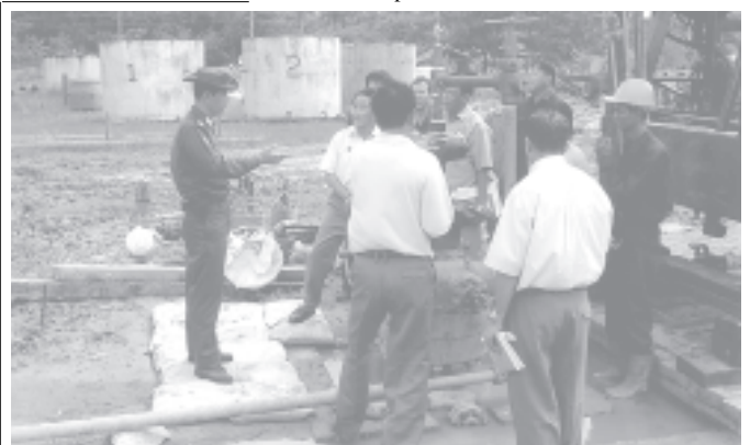
Deputy Minister Brig-Gen Than Htay inspects preparation for repairing of Well No 10 in the Nyaungdon Oil field. — MOE
