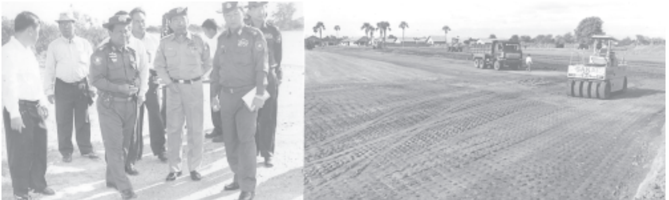
Lt-Gen Ye Myint inspects measures being taken for earth work by the use of heavy machinery at worksite of NyaungU Airport. — MNA
