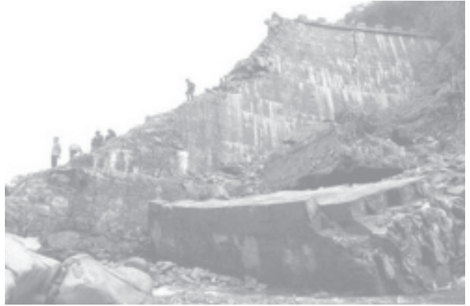
Chinese villagers check the site of a collapsed reservoir in the Xiaocao township of Yiliang county, southwest China's Yunnan Province, on 22 July, 2005.—INTERNET
