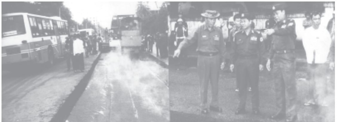
Commander Maj-Gen Myint Swe and Mayor Brig-Gen Aung Thein Lin inspect resurfacing of Strand Road in Kyimyindine. — YGN COMMAND
