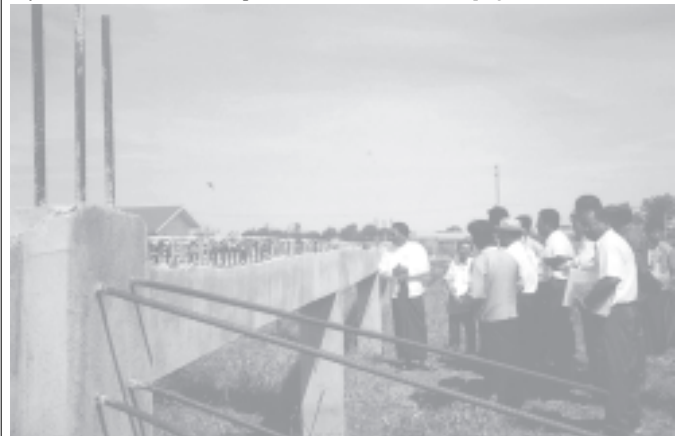
Minister for Industry-1 U Aung Thuang oversees construction of Textile Factory (Myittha) in Myittha.— INDUSTRY-1
