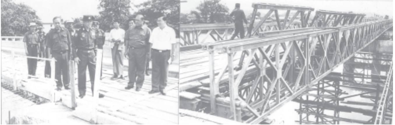
Lt-Gen Khin Maung Than inspects progress in construction of Kaingshay Bridge on Taungup-Kyaukpadaung Road.— MNA
