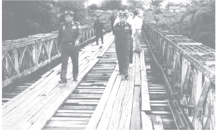
Lt-Gen Ye Myint inspects maintenance of Tabetyan bailey bridge crossing Tabet Creek.
