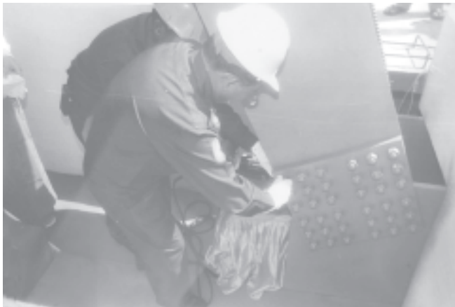
Minister Maj-Gen Saw Tun fixes a nut to complete the work of main frame of Pyapon Bridge in Pyapon township in Ayeyawady Division. (CONSTRUCTION)
