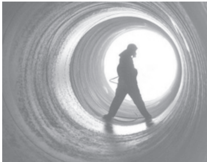
A Chinese worker sprays antiseptic in a pipe with a diameter of 2.6 m (8.5 feet) at a drinking water project in Ningbo in east China's Zhejiang Province on 21 June, 2005. —INTERNET
