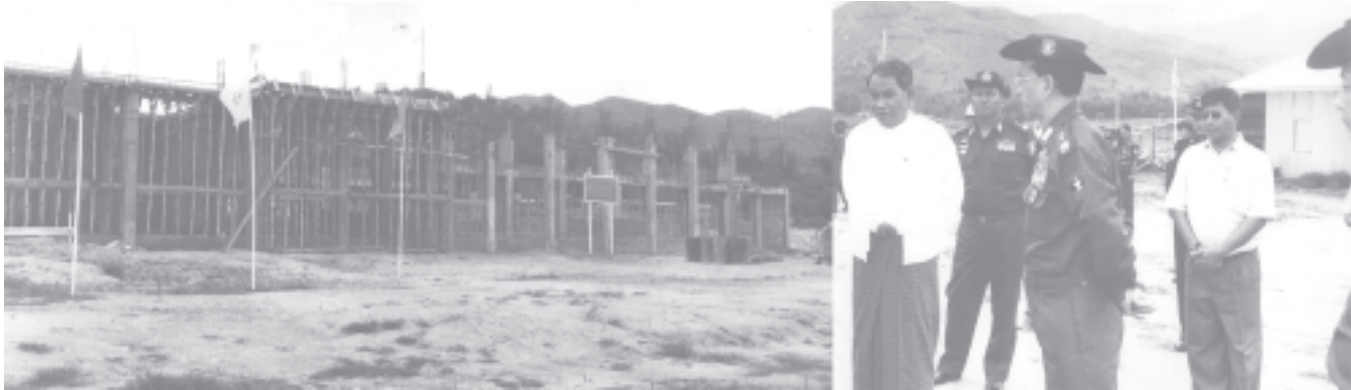
Secretary-1 Lt-Gen Thein Sein inspects construction of two-storey Kengtung Degree College.— MNA
