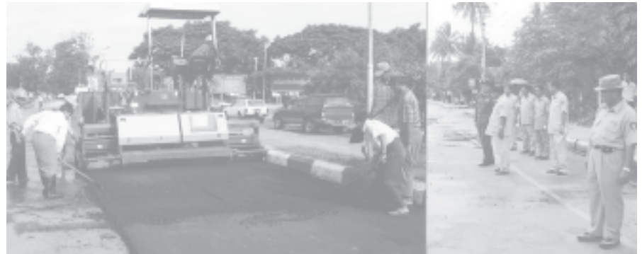
Minister Col Thein Nyunt inspects repaving of Shwemawdaw Pagoda Road in Bago.—DAD
