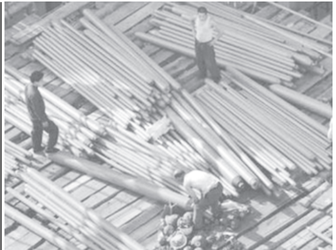
Chinese workers unload steel bars at a construction site in Beijing on 14 June, 2005. — INTERNET
