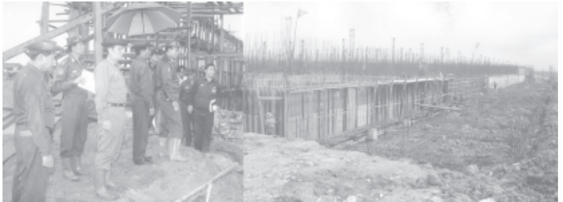
Mayor Brig-Gen Aung Thein Lin inspects Yangon City water supply project (Ngamoeyeik). — YCDC
